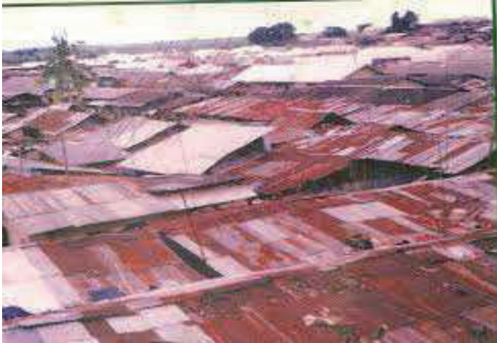
Figure 2.7: Corroded roofing sheets of Niger Delta community due to gas flaring
